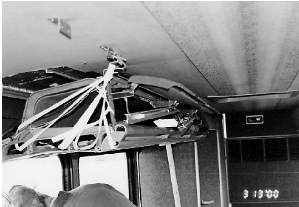
OVERHEAD STORAGE AND LIGHT COMPARTMENT HAS FALLEN DOWN (7,542 TEST MILES)
