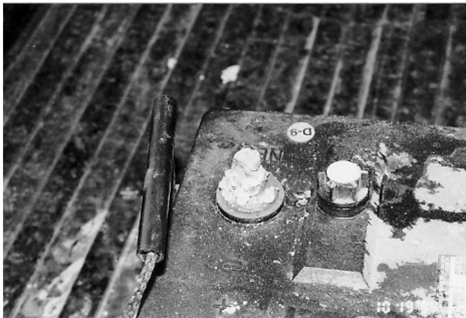
THE NEGATIVE TERMINAL ON THE RIGHT BATTERY IS PITTED (1,725 TEST MILES)
