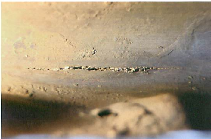
FIGURE 9 —Crack revealed on the inside of a boiler after axial sectioning.
