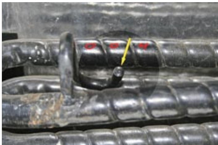
FIGURE 8—Shown is the still intact relief plug of a Norcold N621 refrigerator unit which is located at the top of the absorber coils.
