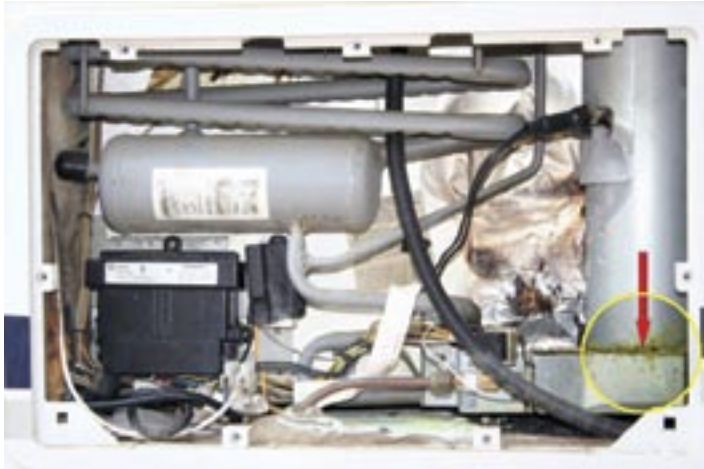
FIGURE 3 —Rear view of a refrigerator in an RV after the refrigerator access panel was removed. Note the yellow residue on the galvanized steel sheet metal and below the incoming propane gas line.
