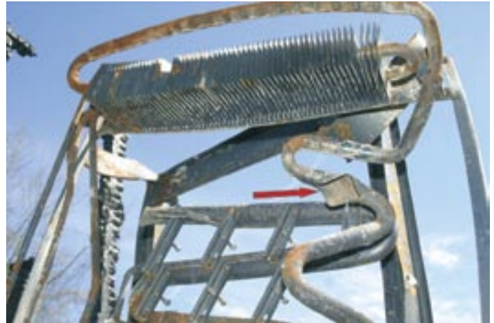
FIGURE 5 —Rupture of the cooling unit involved in a complete RV burn. This unit had maintained pressure up until the point where a fire weakened an area of the cooling unit sufficiently to yield catastrophic failure.
